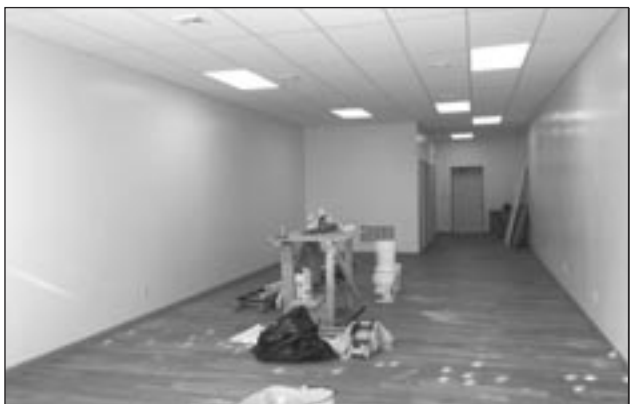
An interior picture of renovations at 164 W. Main St. in Bradford. Photo by Angie Stange.
