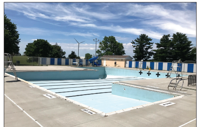
Problems with a broken vent cover have caused the unfortunate closure of the Galva swimming pool during a very warm June. The pool may not open this year. Photo by Carol Townsend.
