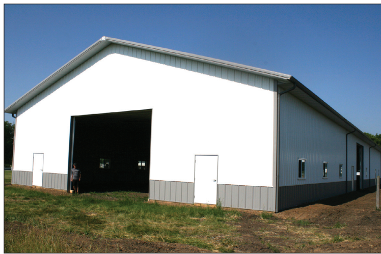
With the main structure up, inside work is ongoing to complete a new exhibition hall for the Stark County Junior Fair in Wyoming. Junior Fair representative Jim Kinsella stands in the doorway. Photo by John A. Ballentine.
