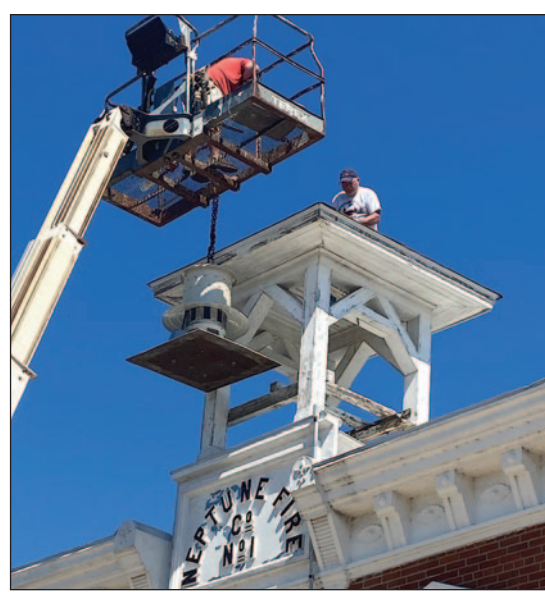
Elmwood electrician Jeremy Martin of Tannock Electric (left) and Elmwood contractor Dave Hall installed a new siren on top of Elmwood City Hall Tuesday morning. The old siren – or “noon whistle” – was damaged in a storm and had been silent for months. The City of Elmwood and the Elmwood Fire Department each agreed to pay for half of the cost of the new siren, which was $4,728. The siren could be heard several times across town on Tuesday after it was installed. Photo by Jeff Lampe.
