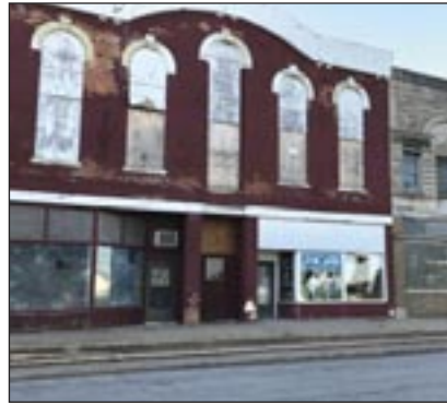
Pictured are the back (top) and front of the former ceramic buildings on Main Street downtown that the city of Galva purchased recently.
