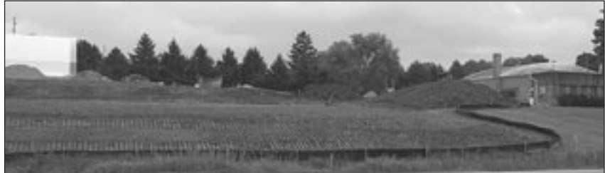
Construction work for Toulon's new Dollar General store has started with the removal of a large tree and groundwork being done for the new building located at Stark County's highway department property in Toulon. Photo by John A. Ballentine.
