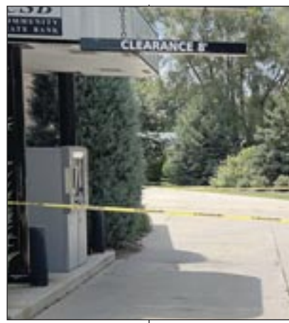
Pictured is the lane which remains closed at Community State Bank in Galva after a truck left ruts in the grass at the right pulling the ATM from the building. The ATM and stolen truck were left near the Galva Cemetery, which is located south of Galva in Knox County. Photo by Carol Townsend.
