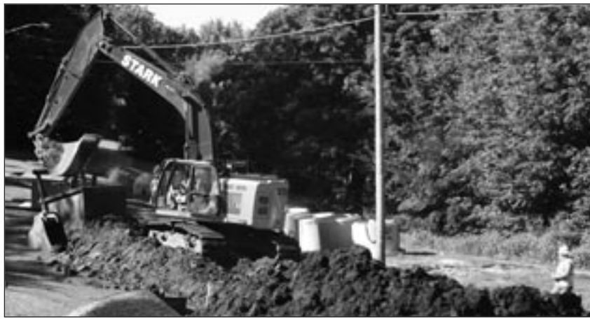
After more than 1 1/2 years, Stark Excavating is moving dirt for the new sewer lift station site at Prairie and Whittaker Streets in Toulon. Photo by John A. Ballentine.
