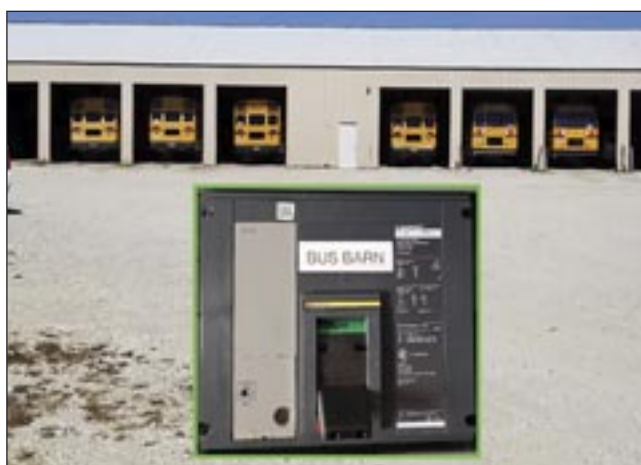
The Williamsfield bus barn will house a fleet of electric-powered vehicles next year thanks to a $2.6 million federal grant. Buses will also provide energy storage once the bus barn switch is flipped and all buildings are connected to a micro grid. Photo/graphic by Tim
