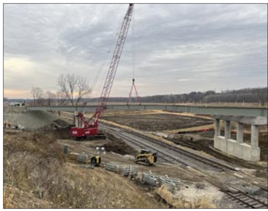
Crews worked Tuesday morning to set the final steel beams on the new Illinois Route 8 bridge south-east of Edwards. Photo by Doug Whitney.
