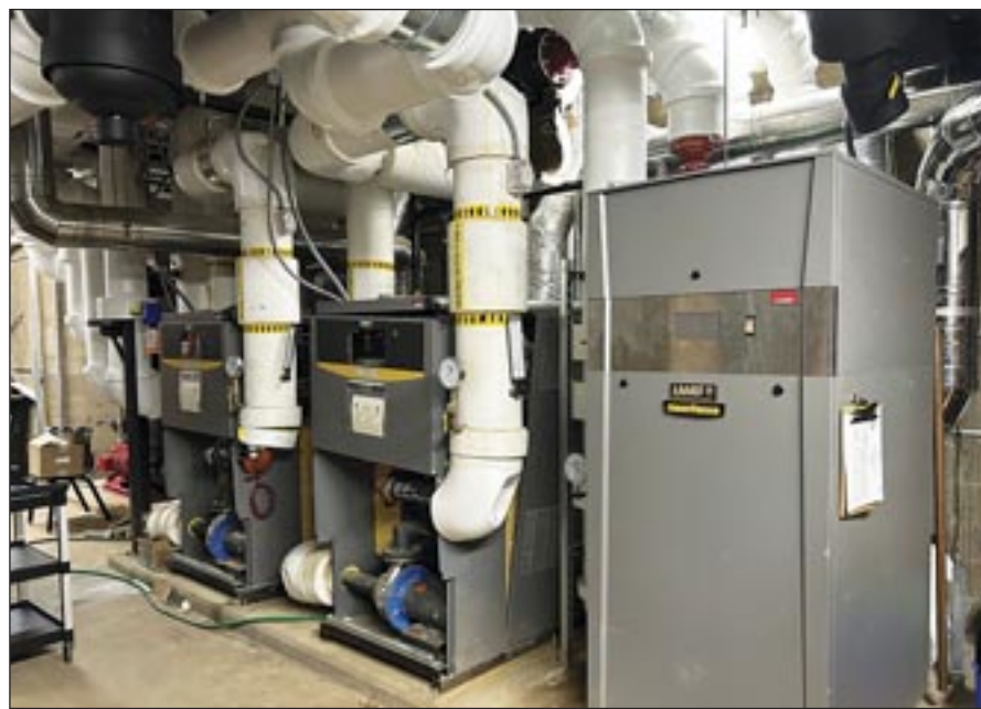
At left are two boilers that have failed in the Elmwood schools building. The boilers were installed in 2016. At right is a boiler installed last fall that is still running.
