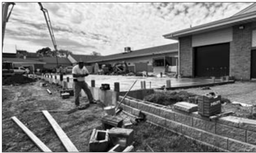
The concrete floor of the Elmwood School District’s new Claude W. Keefer Industrial Arts building was nearing completion Tuesday afternoon. Work on the building is expected to be completed in time for the start of the 2023-24 school year. Photo by Jeff Lampe.
