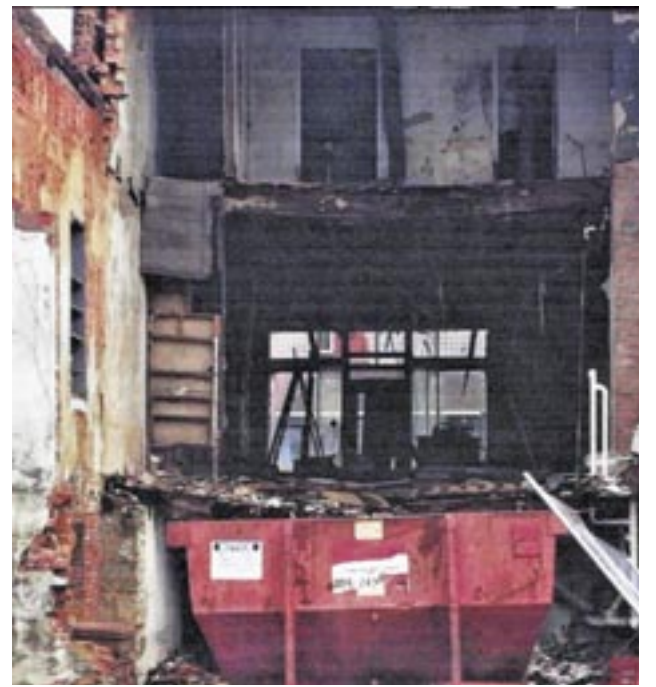
The space at 54 E. Fort St. in Farmington has been transformed from its state prior to renovation. Photo by Dave Giagnoni.
