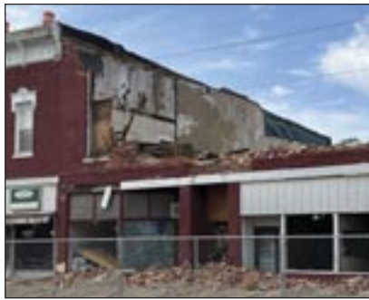
Demolition work on Front Street in Galva has been halted. Photo by Carol Townsend.
