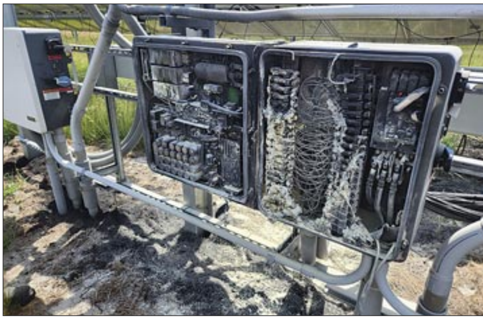
A fire June 9 damaged the fuse panel and inverter panel at a solar farm located on Illinois Route 116. The fire spread to nearby grass. Photo courtesy of the Farmington Community Fire Protection District.
