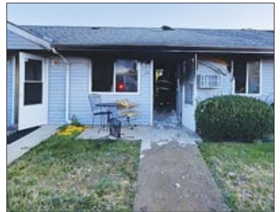
Fire damaged the Farmington Manor apartment complex at 700 E. Court St. on Sept. 14. For details, visit Page 8. Photo courtesy of the Farmington Fire Department.
