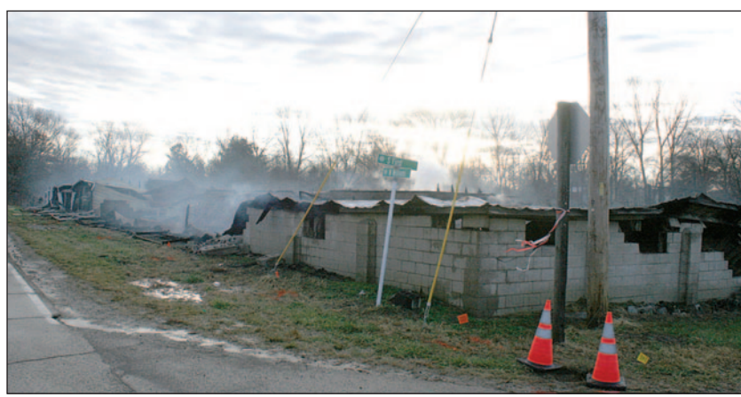
An early-morning fire destroyed the Wyoming Horse Sale Barn on Dec. 9. One full-sized horse, two miniature horses and a donkey perished in the fire. Photo by John A. Ballentine.
