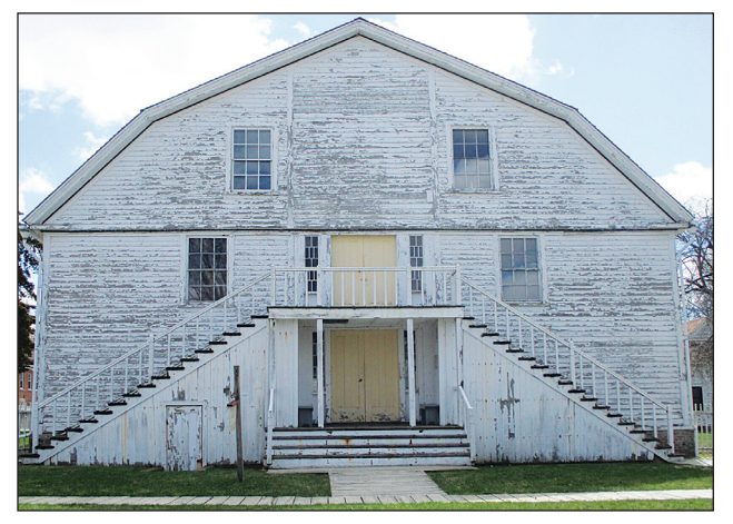
Peeling paint is among the issues facing the Bishop Hill Colony Church, listed as one of 10 of the most endangered historic places in Illinois by Illinois Landmarks. Photo courtesy of the Bishop Hill Heritage Association.
