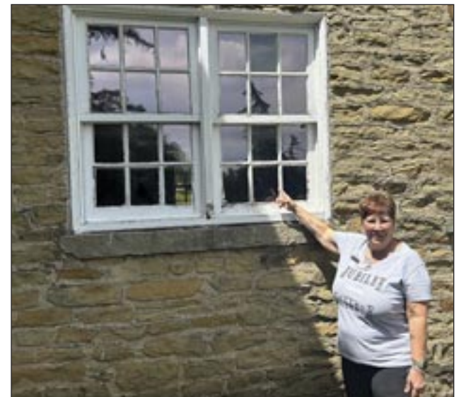
Lonye Gilles points to one of several deteriorating windows at the Jubilee College State Historic Site. Photo by Jeff Lampe.
