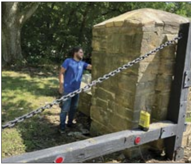
Work is underway to restore the stone gates at the old entrance to Jubilee College State Park. The Citizens Committee to Preserve Jubilee College is funding the work, which is expected to cost $3,600 per gate. One gate will be done this year and another is scheduled to be completed next spring. Photo by Lisa Sandall.
