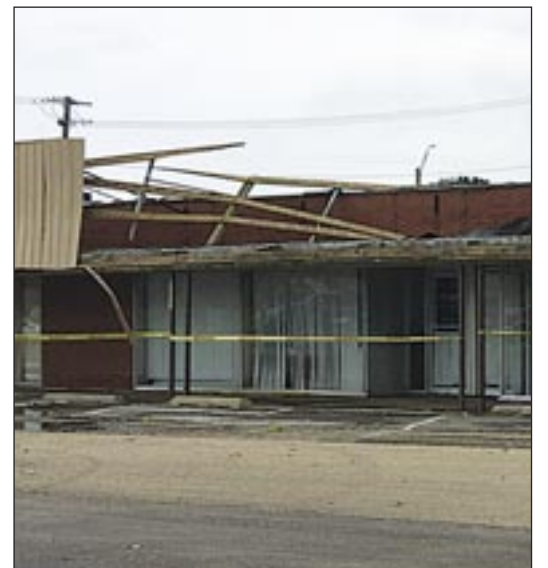
The facade at Midland Plaza in Kewanee suffered extensive damage during the July 16 storms that resulted in Henry County being declared a state disaster area late last week.
