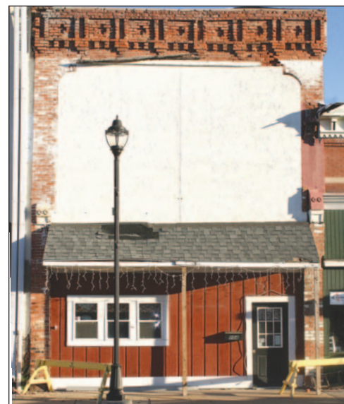
Pictured above is the unstable building facade at 104 E. Williams St. in Wyoming. Photo by John A. Ballentine.
