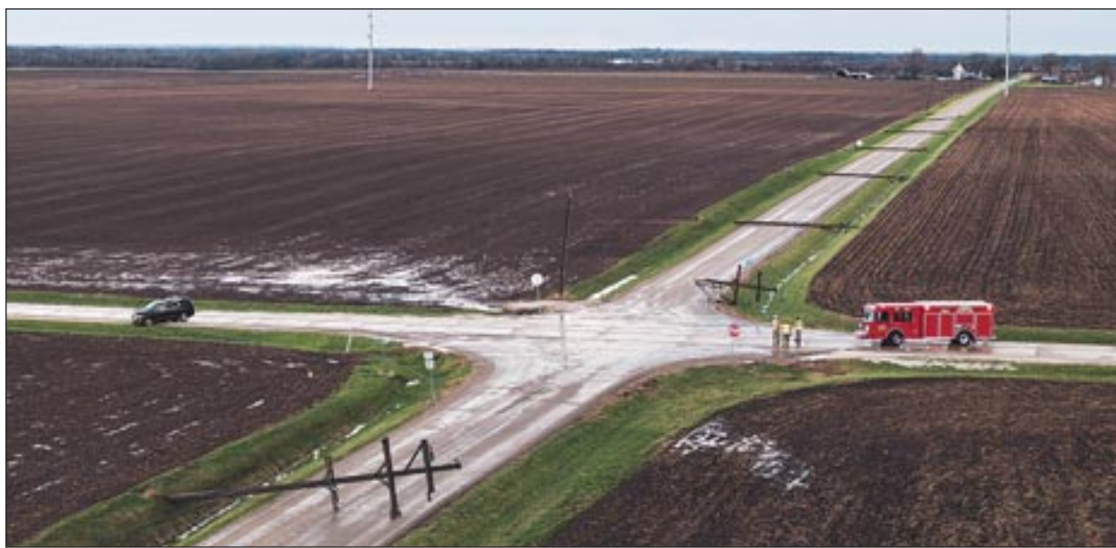
Power poles were downed by a tornado April 2 along Elmore Road and U.S. Route 150 southwest of Laura. A vehicle, pictured above, was stranded on the scene after it was entangled with the wires. Photo by Andrew Pritchard of chambanaweather.com. Below, the wind damaged a shed on the farm of Les Potts, northwest of Yates City.
