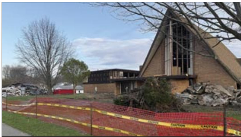
Demolition of the former St. Matthew Roman Catholic Church at 156 E. Vernon St. in Farmington is moving forward. All that is left of the parsonage is the pile of rubble to the left in this picture. Demolition stems from the Diocese of Peoria's decision in 2024 to close the church and merge the parish with St. Mary of Canton. Once demolition is completed, the vacant lot will be for sale. Photo by Jeff Lampe.
