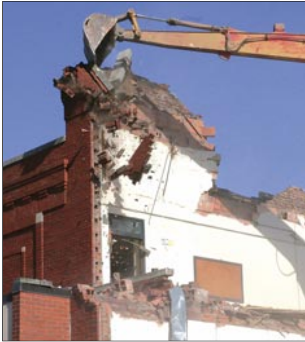
An excavator tears down a brick wall of the old Farmington Junior High School. Photo by Dave Giagnoni.
